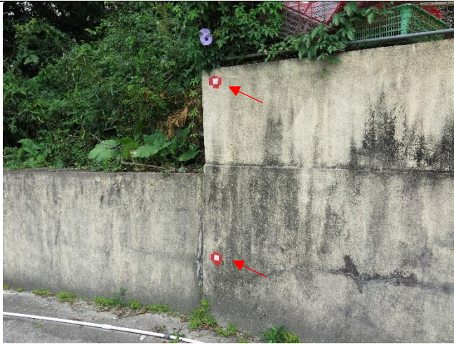
Photo 2: Reflective targets for settlement monitoring were installed on the fence wall at NP-10.
