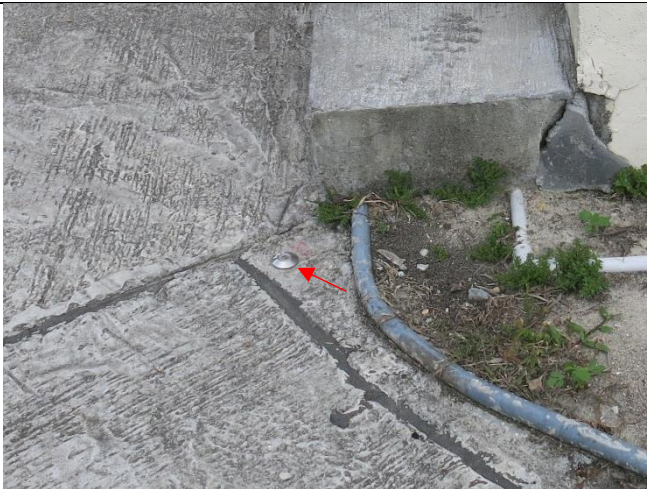
Photo 5: Ground settlement marker for settlement monitoring was installed at the entrance of NP-11.
