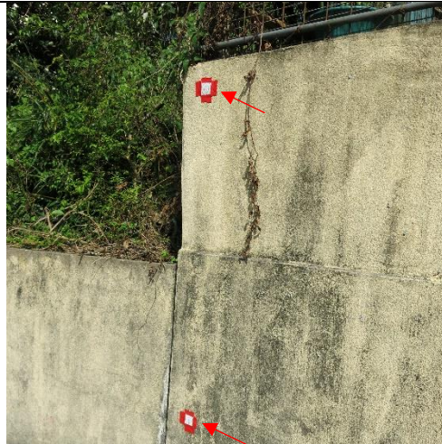
Photo 2: Reflective targets for settlement monitoring were installed on the fence wall at NP-10.
