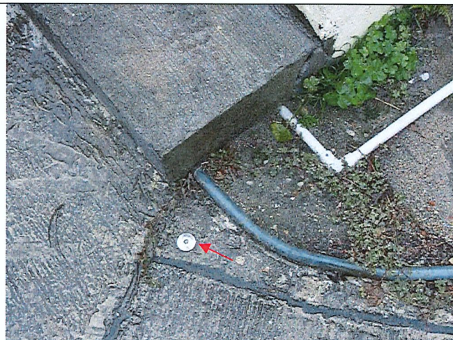
Photo 5: Ground settlement marker for settlement monitoring was installed at the entrance of NP-11.
