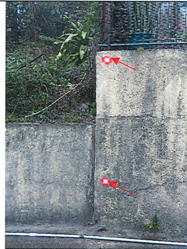
Photo 2: Reflective targets for settlement monitoring were installed on the fence wall at NP-10.
