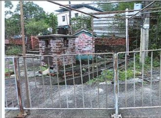
Photo 12: The notice at NP-26 was found missing. Replacement is required.
