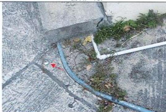
Photo 5: Ground settlement marker for settlement monitoring was installed at the entrance of NP-11.
