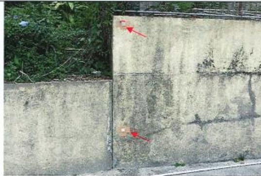
Photo 2: Reflective targets for settlement monitoring were installed on the fence wall at NP-10.
