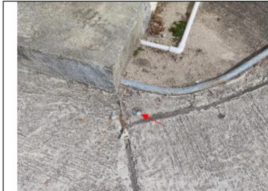
Photo 7: Ground settlement marker for settlement monitoring was installed at the entrance of NP-11.
