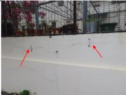
Photo 5: Tell-tales for crack monitoring were installed on the fence wall at NP-10.
