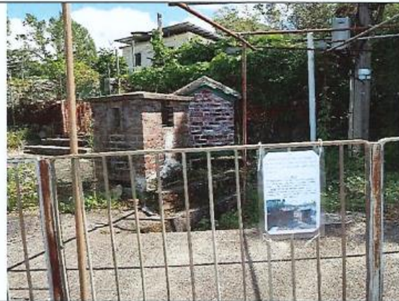
Photo 14: A warning notice was placed near NP-26.
