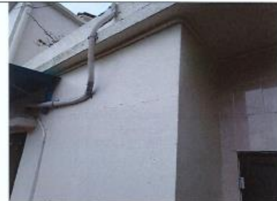
Photo 3: Tell-tales (TT1 & TT2) for crack monitoring were removed by the owner at NP-10 due to renovation works; Crack was repaired.
