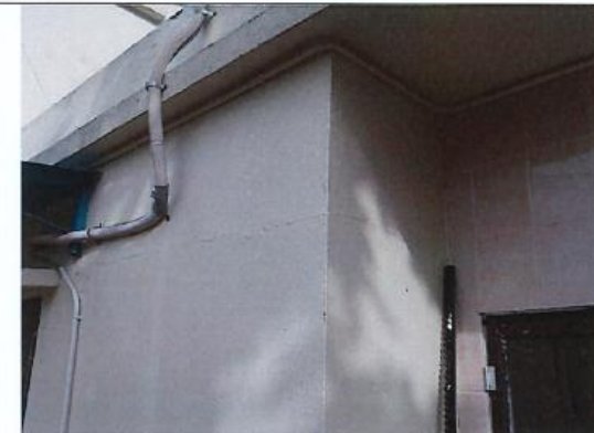
Photo 3: Tell-tales (TT1 & TT2) for crack monitoring were removed by the owner at NP-10 due to renovation works; Crack was repaired.
