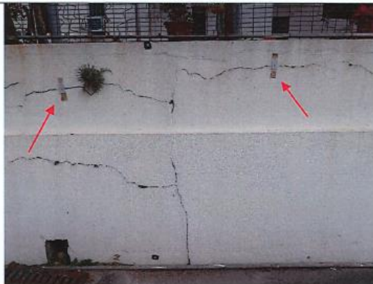
Photo 5: Tell-tales for crack monitoring were installed on the fence wall at NP-10.
