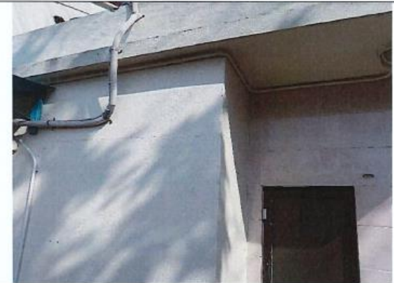
Photo 3: Tell-tales (TT1 & TT2) for crack monitoring were removed by the owner at NP-10 due to renovation works; Crack was repaired.
