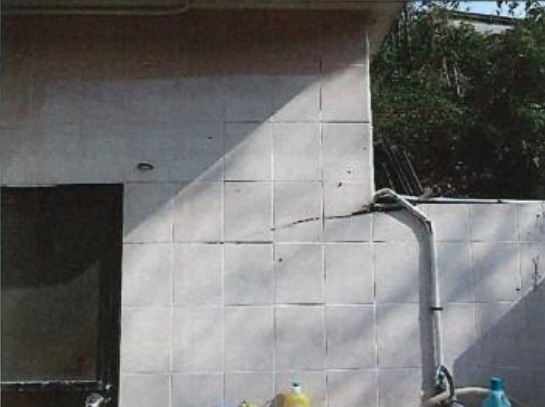
Photo 4: Renovation works were done at NP-10 except for the walls in Kitchen & Lavatory at the time of inspection.
