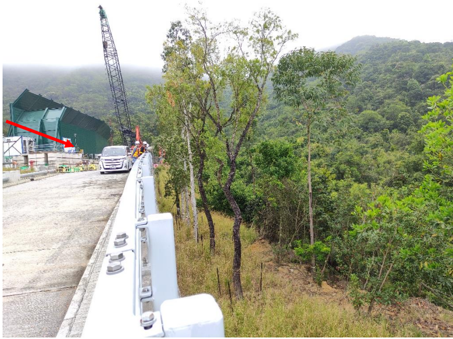
Photo B.15: Construction activities observed during the monitoring on 17 Mar 2023 but not adjacent to the receptor site.
