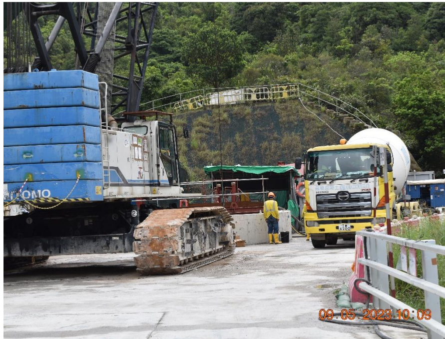
Photo B.9: Construction activities observed during the monitoring on 09 May 2023 but not adjacent to the receptor site.
