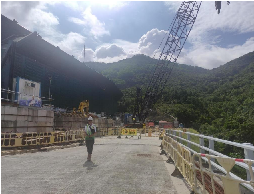
Photo B.9: Construction activities observed during the monitoring on 08 August 2023 but not adjacent to the receptor site.
