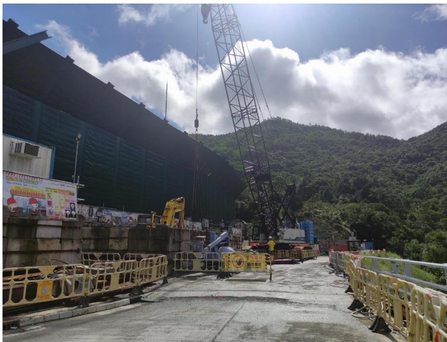
Photo B.10: Construction activities observed during the monitoring on 12 September 2023 but not adjacent to the receptor site.
