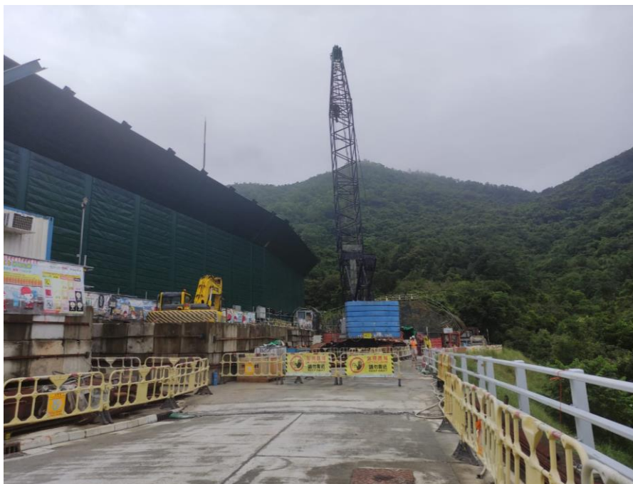
Photo B.10: Construction activities observed during the monitoring on 10 October 2023 but not adjacent to the receptor site.
