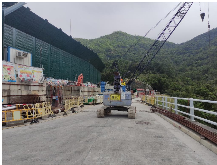
Photo B.10: Construction activities observed during the monitoring on 08 November 2023 but not adjacent to the receptor site.
