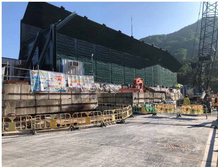
Photo B.10: Construction activities observed during the monitoring on 05 December 2023 but not adjacent to the receptor site.
