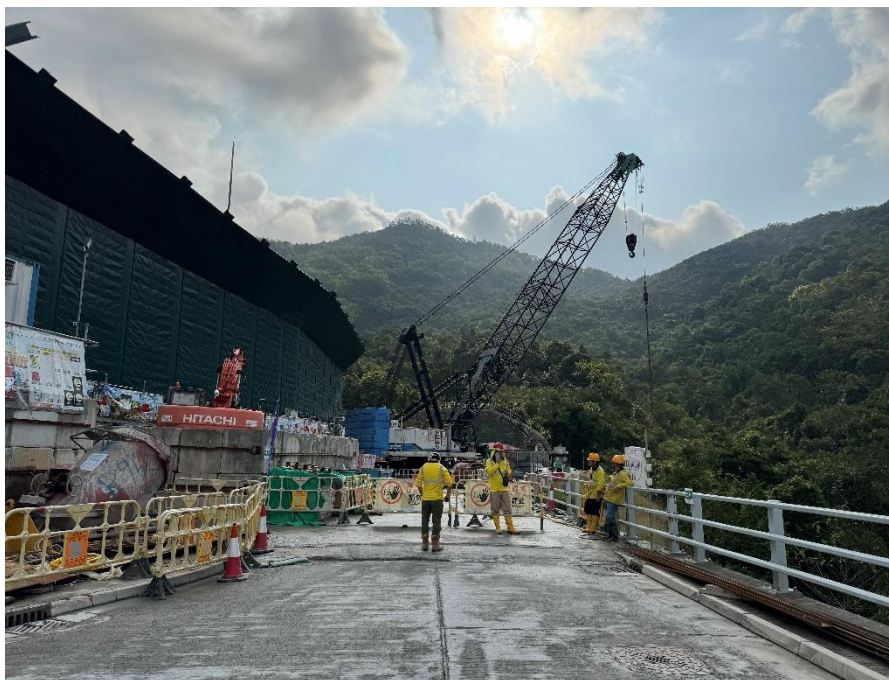
Photo B.10: Construction activities observed during the monitoring on 05 March 2024 but not adjacent to the receptor site.
