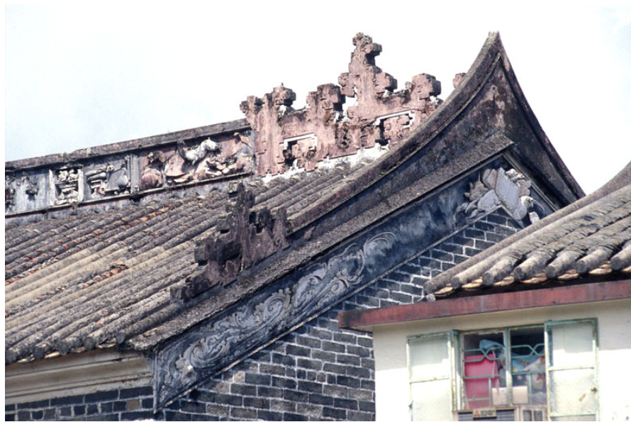
Plate 3 Stucco mouldings on ridges and gables walls are fading.
