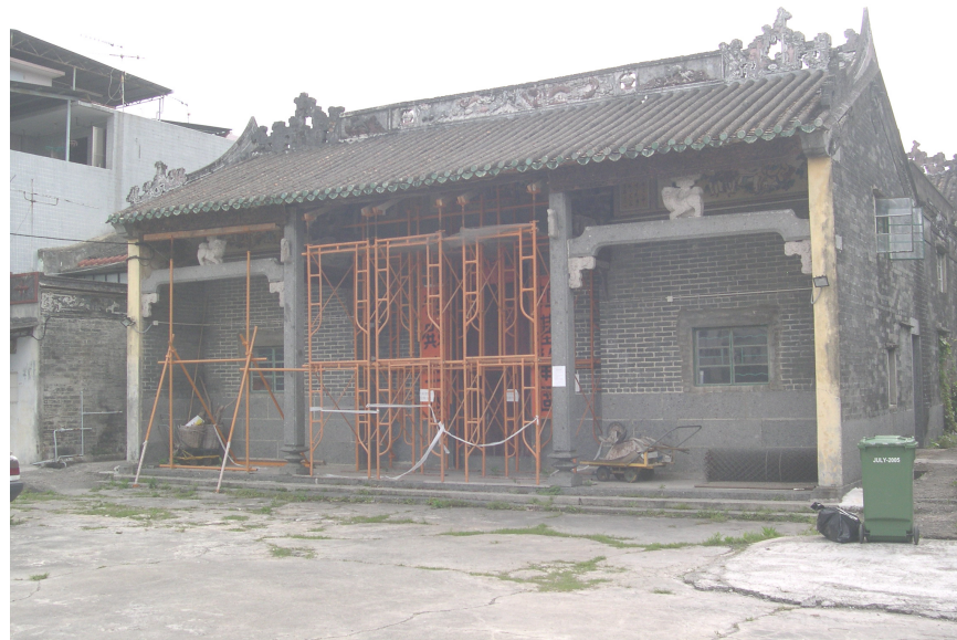
Plate 1 The front elevation of the Chik Kwai Study Hall. Temporary propping has been erected by AMO.
