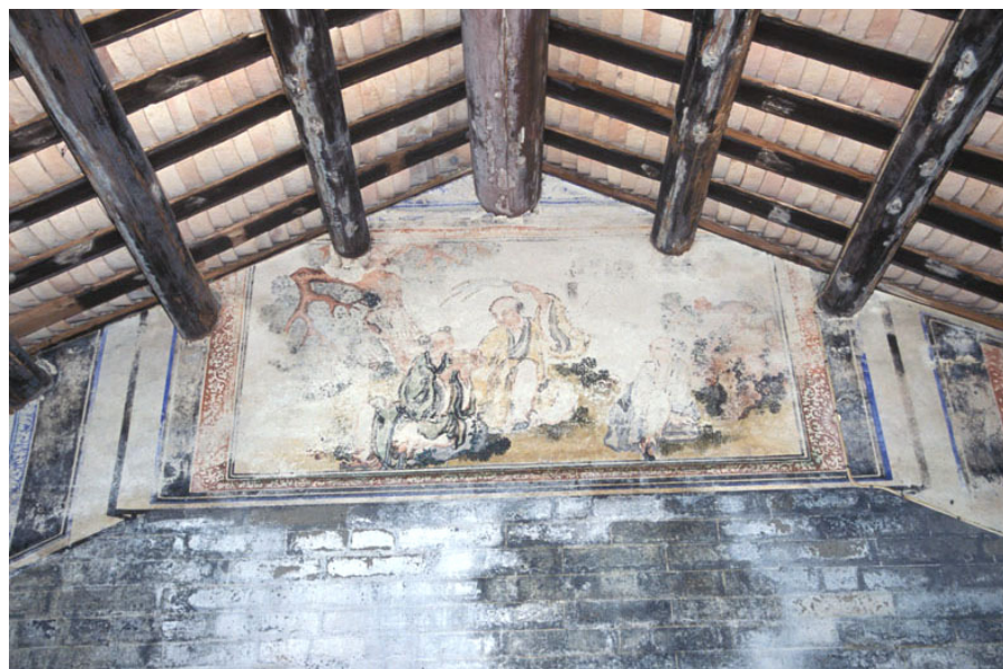
Plate 4 Conservation treatment to historic murals throughout the building is required.
