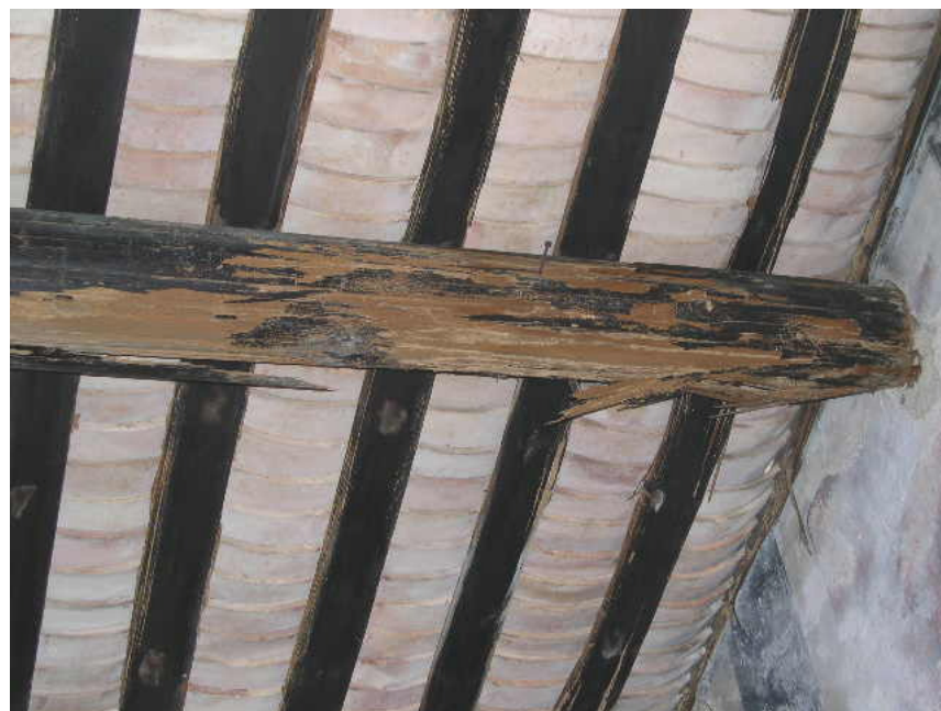
Plate 2 Purlins in the Study Hall have been infested by termite.
