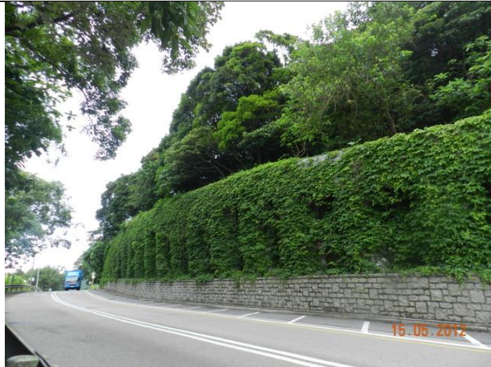
VP14 – Located to the southeast of the Works Area and opposite to the proposed flexible barriers in the woodland
