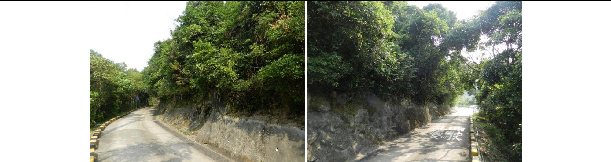
VP1 – Located next to Tai Wan Tau Road and next to Lamppost # EB9732
