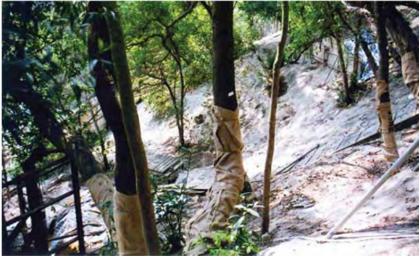
Protective wrapping around tree trunks (Source: GEO Publication No. 1/2011)
