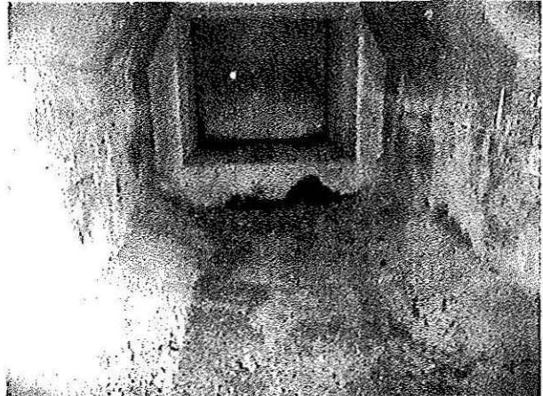
Photo 2. General view for the interior of Incinerator No. 2. Photo taken at Incinerator Room, LG 2/F, Main Block.
