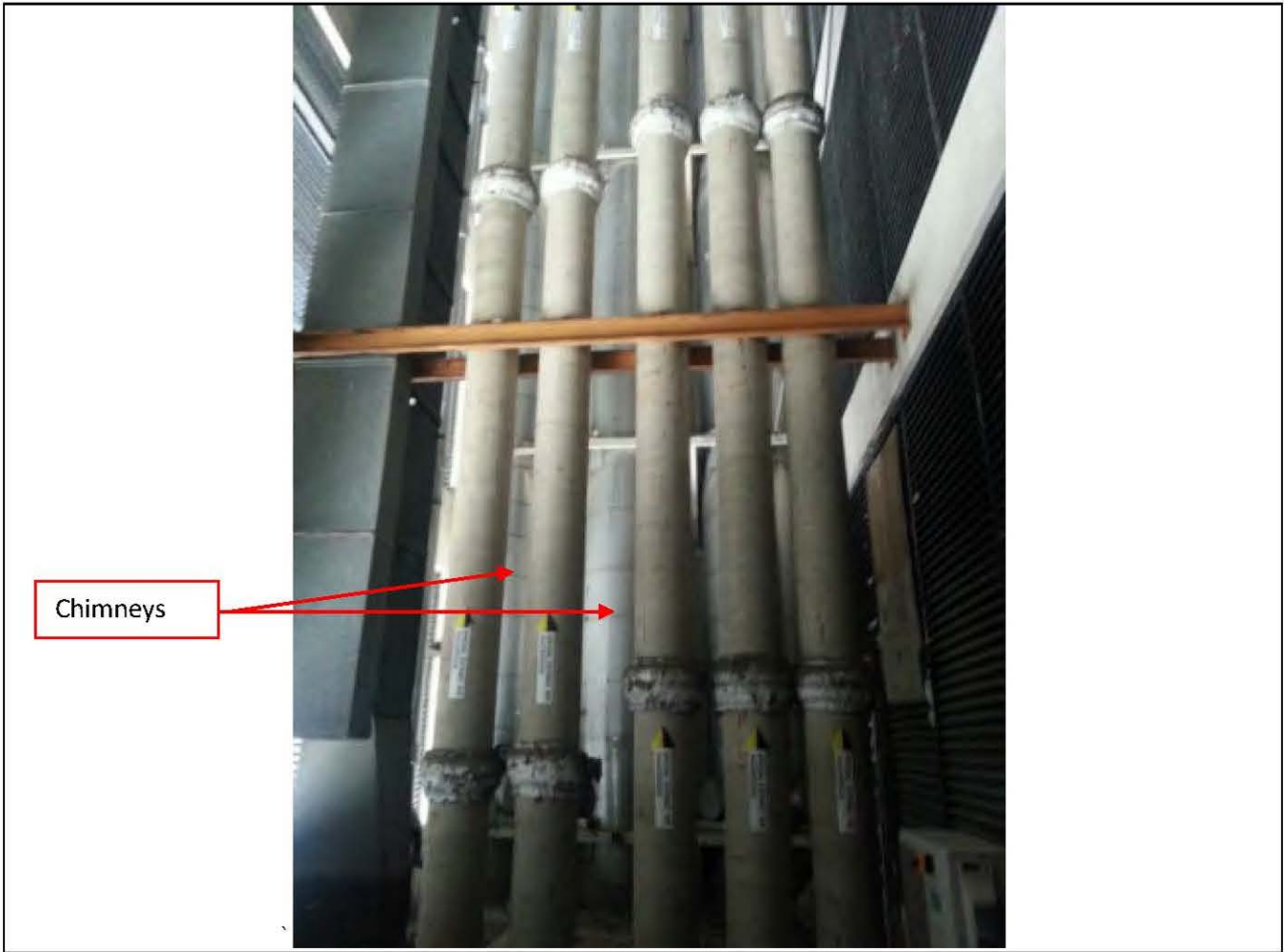
Chimneys (only 2 chimneys for incinerators)
