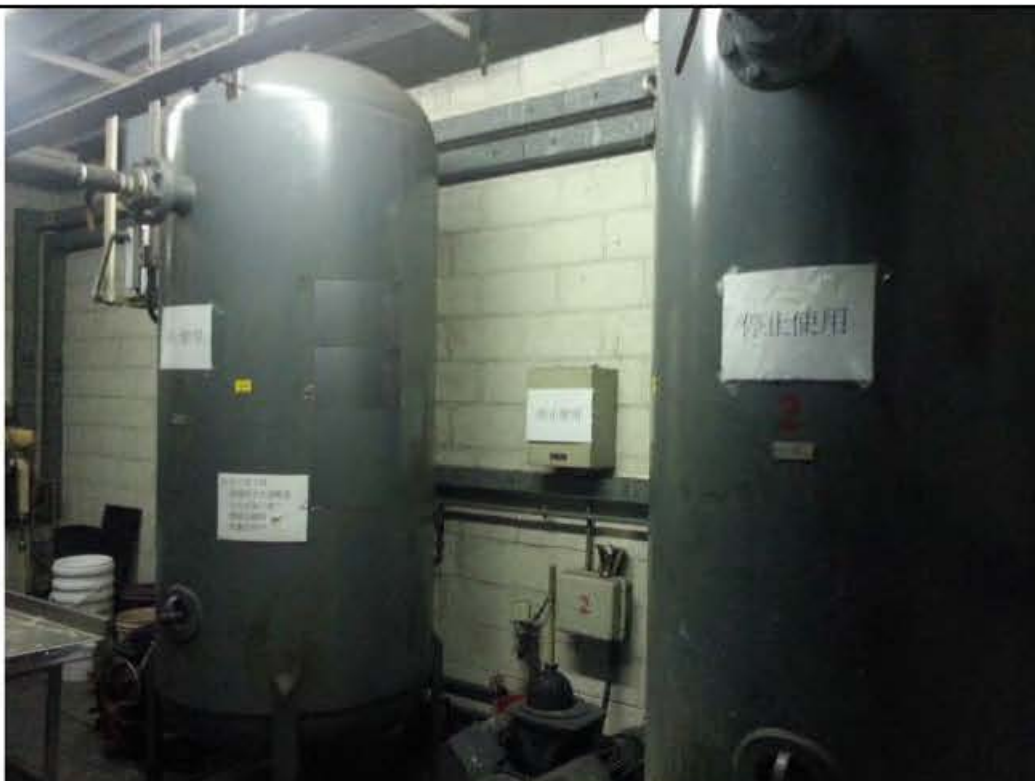
Air receivers and compressors
