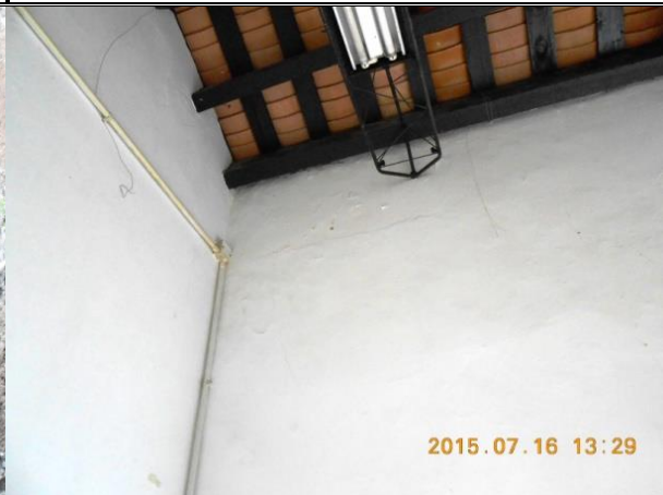
4) Cracks on the ceiling inside the Annex Block
