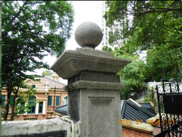
2) Dislocated upper compartment of the western gate post by Caine Lane
