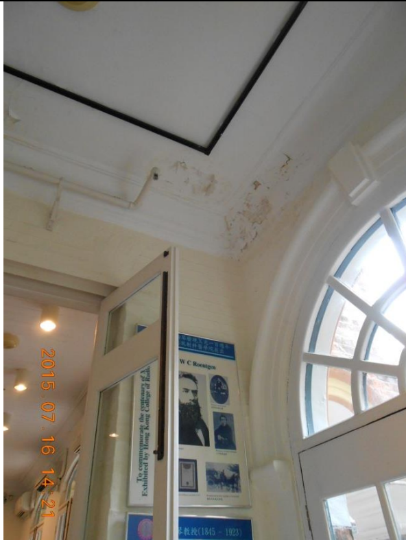
1) Cracks on the ceiling on the first floor
