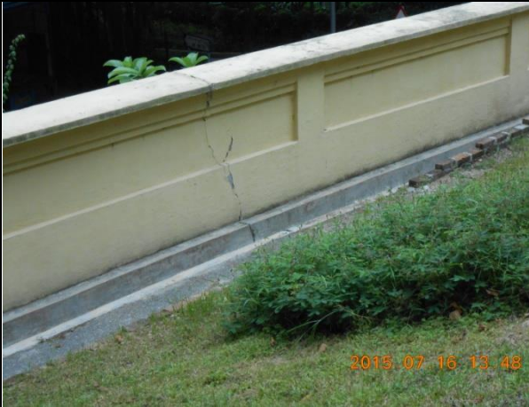
1) Crack on the fence wall next to Feature No. 11SW-A/R218, south to the lawn of the Main Building of the Hong Kong Museum of Medical Sciences
