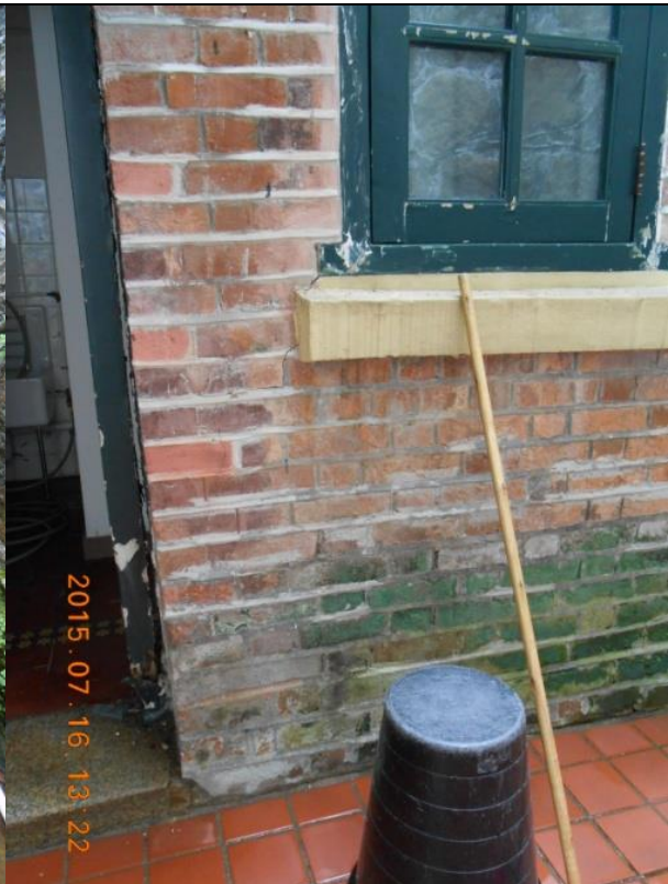
2) Cracks on the external brick wall of the Annex Block
