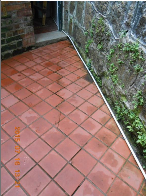
1) Settlement cracks in front of the eastern corner of the area enclosed by the Annex Block and Feature No. 11SW-A/R94
