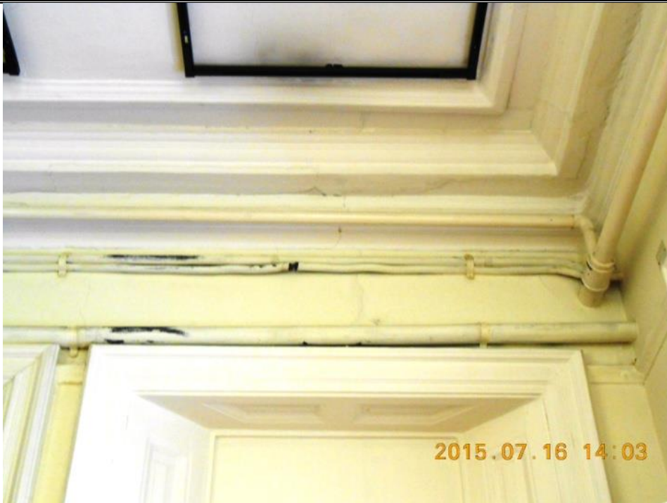
3) Cracks on wall above the door on the ground floor
