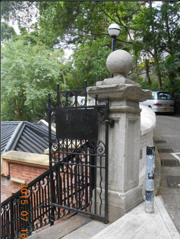
3) Eroded/damaged upper compartment of the eastern gate post by Caine Lane
