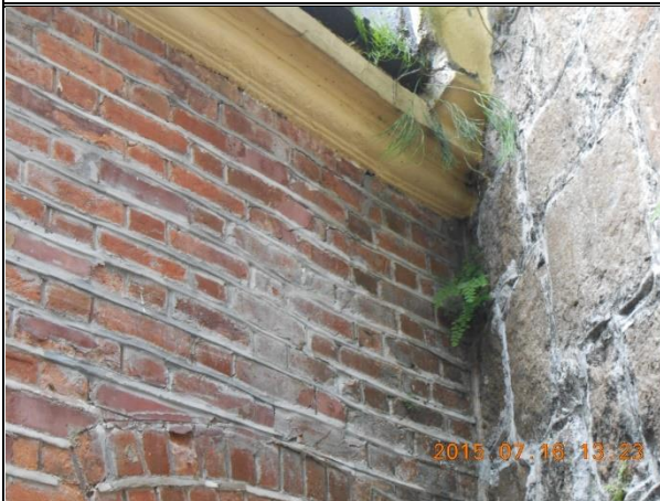
3) Wall cracks on the Annex Block adjacent to Feature No. 11SW-A/R94
