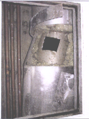
The vertical incinerator flue pipe section on the lower ground floor has been cut open for inspection
