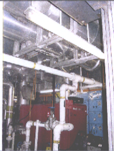
Incinerator flue pipe in the boiler room
