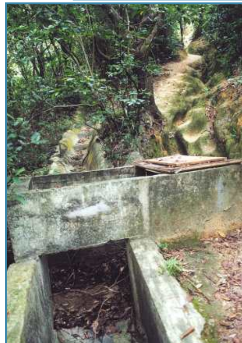
Plate 5 2 nd arm of the drainage channel runs directly up the slope, at right angles to the proposed cable alignment.
