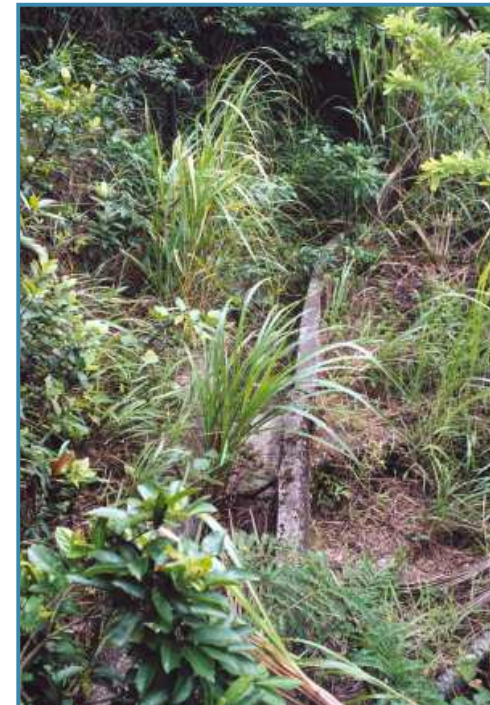
Plate 3 The drainage channel is partly broken at this point midway along the route shared with the cable alignment.
