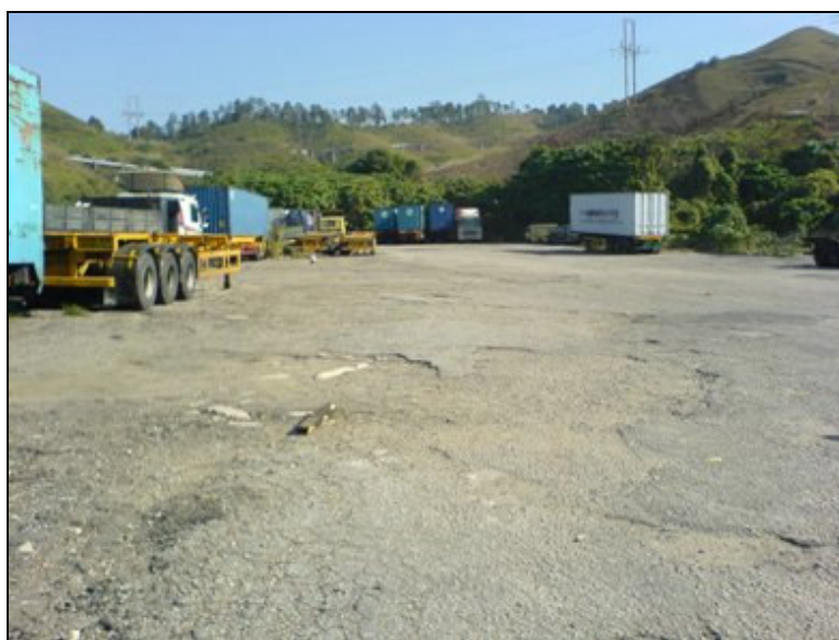
Photograph 3-3 Existing Poor Condition of the Hardstanding within the Site
