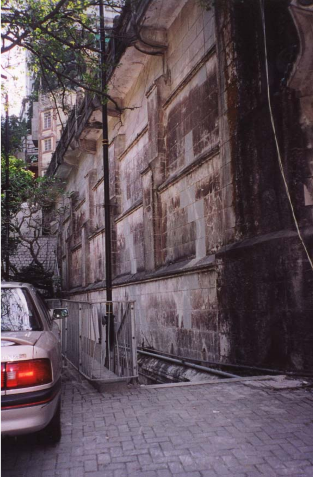
Figure 9.3 View of the Boundary Wall of the Haw Par Mansion (from works area to the east)
