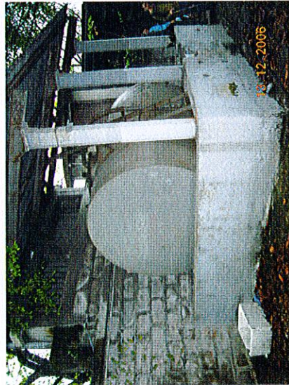
10 - Aboveground Storage Tank (Facing Southwest)
