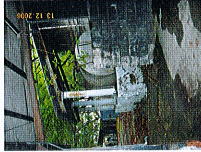
11 - Aboveground Storage Tank (Facing East)
