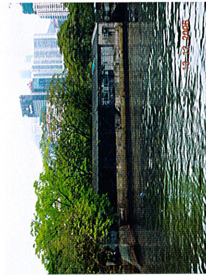
1 - Workshop B and Site Office on Seawall and Thick Concrete (Facing South)
