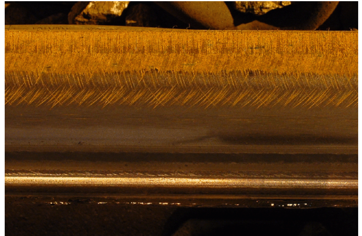
PHOTO 7 RUNNING SURFACE OF HIGH RAIL
