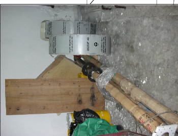
CONTAINERS STORAGE AREA INSIDE THE STANDBY GENERATOR ROOM
