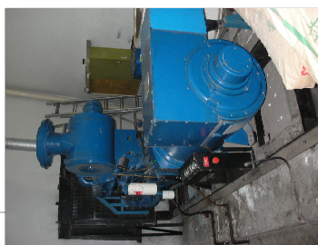
EMERGENCY ELECTRICITY GENERATOR LOCATED AT THE STANDBY GENERATOR ROOM
