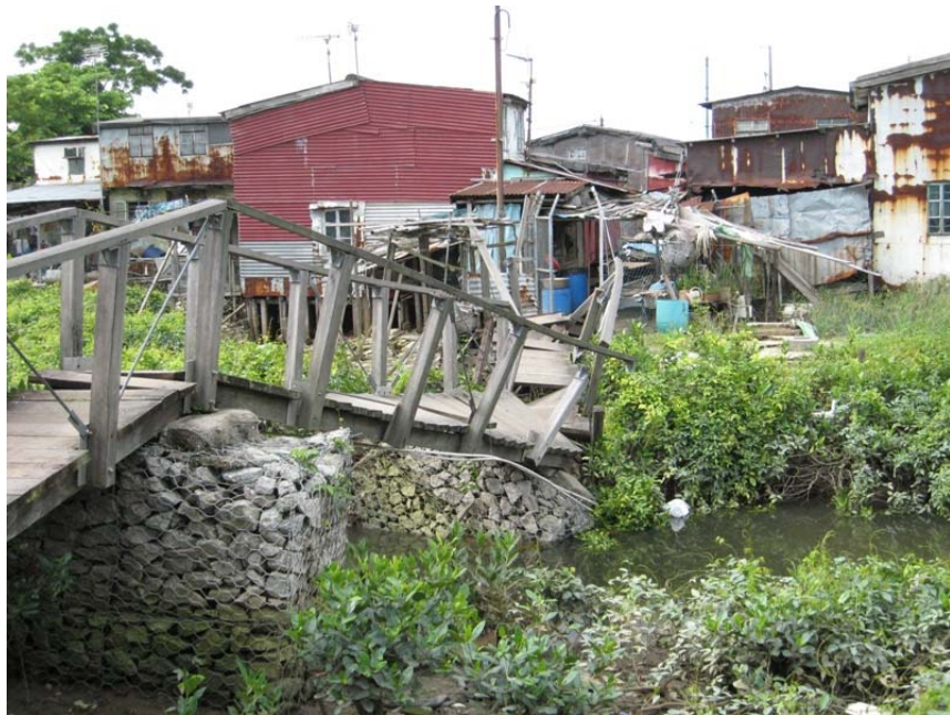
Plate 10 Collapsed footbridge (16 June 2008).
