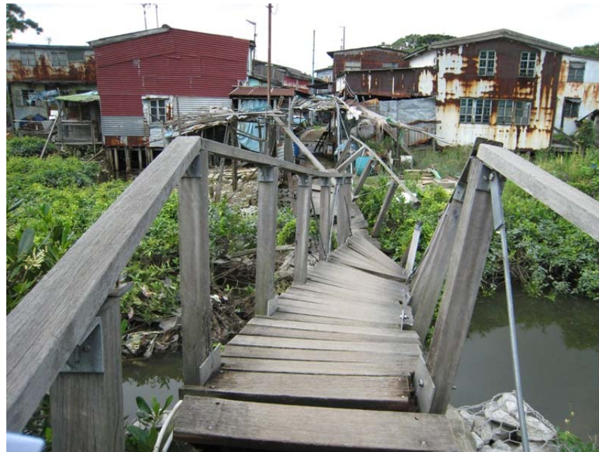
Plate 11 Collapsed footbridge (16 June 2008).
