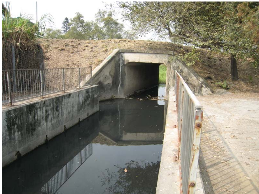
Plate 4 Water from San Hing Tsuen Channel and Fung Kong Tsuen Channel merges and drains into Hang Hau Tsuen stream via a single cell box culvert underneath Deep Bay Road.
