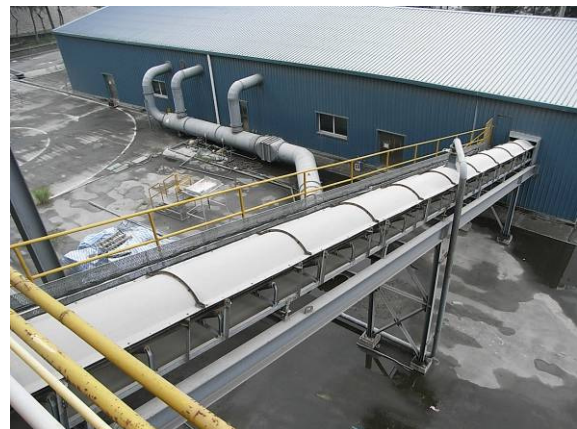
Photo 4 – Conveyor belt connecting the CCPP unit with the material recovery building
