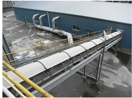
Photo 2 – Conveyor belt connecting the CCPP unit with the material recovery building
