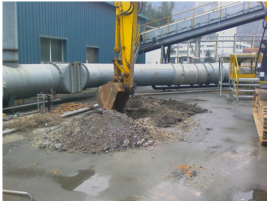
Photo 3 – Breaking of concrete surface at S1/S2
