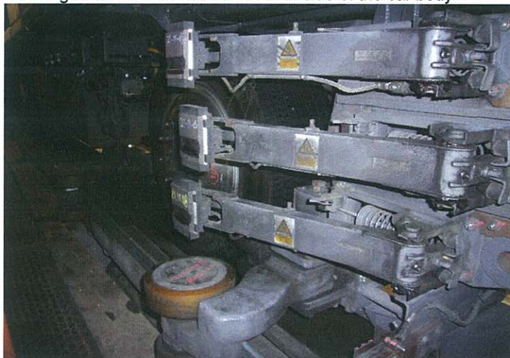
Existing APM - Guide Wheels on both side of the car body
