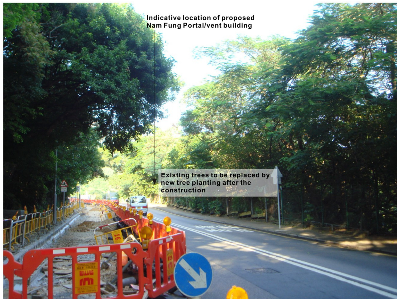
Existing Condition Vantage Point E - View east at Nam Fung Road looking towards the proposed Nam Fung Portal / Vent Building
