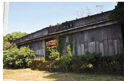
Photo 2 – Corrugated zinc sheet roof and bitumen sheet waterproofing layer at the main entrance
