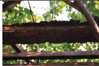
Photo 6– Significant rusting at beam on roof
