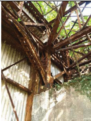
Photo 8 – Corroded and deteriorated steel frame
