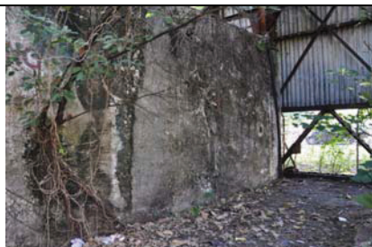
Photo 3 – Mass Concrete side wall with grown vegetation
