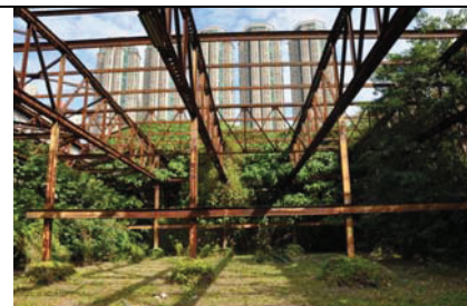
Photo 4 – Significant rusting at beam on roof
