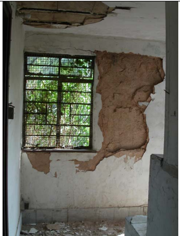
Photo 8 - Spalling and exposed reinforcement at 1/F
