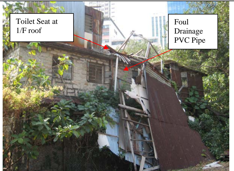
Photo 16 – Toilet Seat & Foul Drainage pipe at 1/F roof
