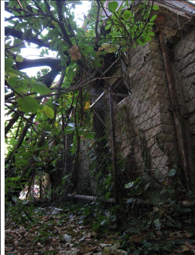
Photo 22 – Tree at North-West side of House near roof of G/F
