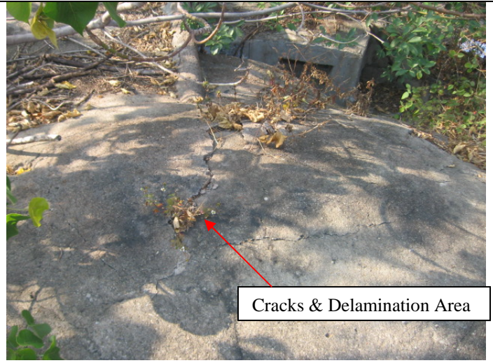
Photo 36 – Delamination at roof top
