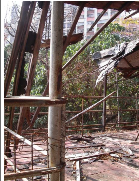
Photo 7 – Part of Shelter has collapsed
