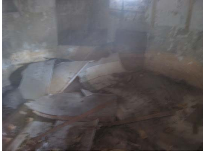
Photo 31 – Some debris, damaged timber boards and rods are found on the floor
