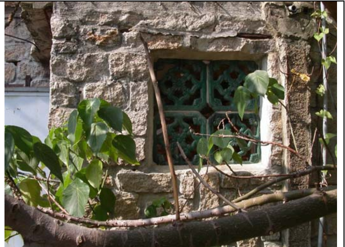
Photo 19 – Greenish Ceramic Window Frame
