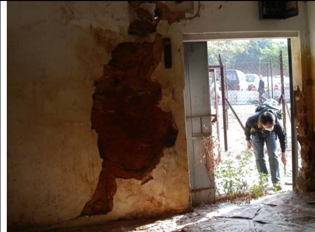
Photo 9 – Poor condition of internal wall
