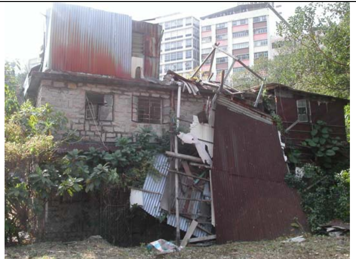
Photo 6 – Part of temporary squatter structure were fallen down to the backyard of Stone House
