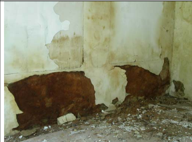
Photo 11 - Loose plaster, timber rods & boards
