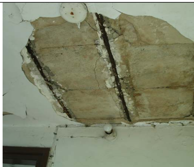
Photo 4 – Rusted Reinforcement under the 1/F Roof
