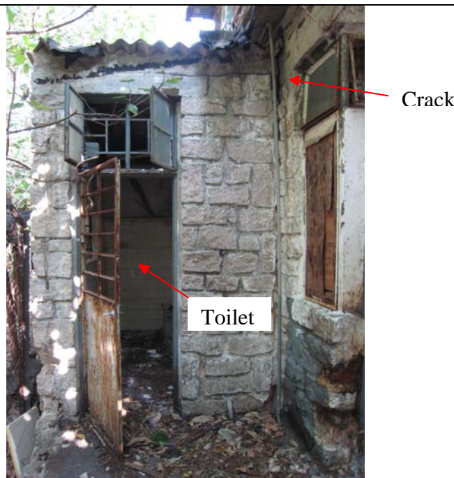
Photo 14 – Crack at G/F Toilet
