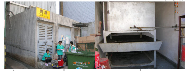
FUEL TANK ROOM AND EMERGENCY GENERATOR ROOM OF THE INTERNATIONAL MAIL CENTRE
