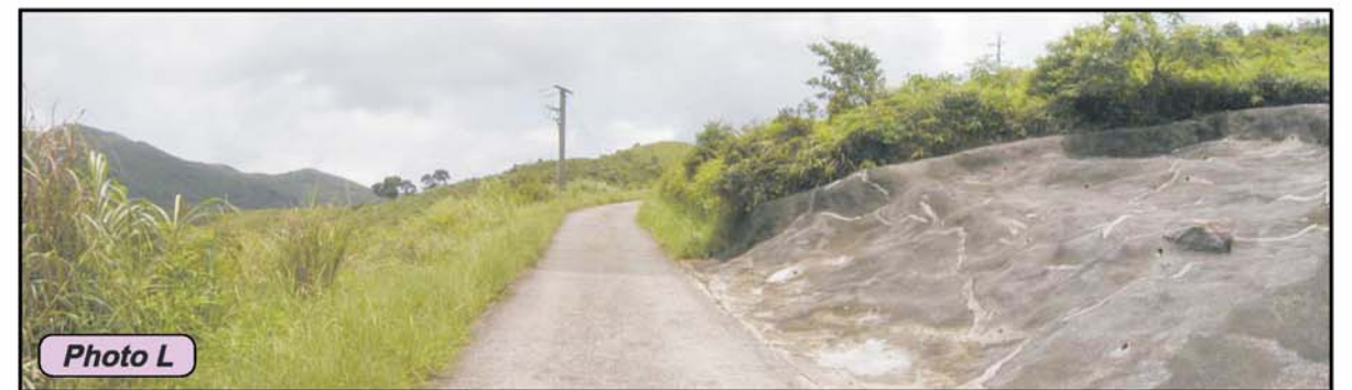
Existing Road Condition at Section 7 - 7
