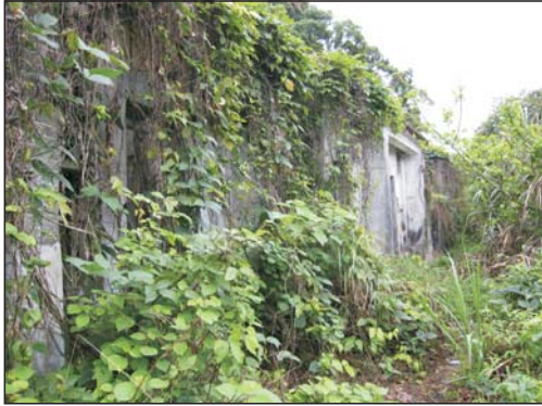
Broken village houses at Lei Uk overgrown with weeds and climbers
