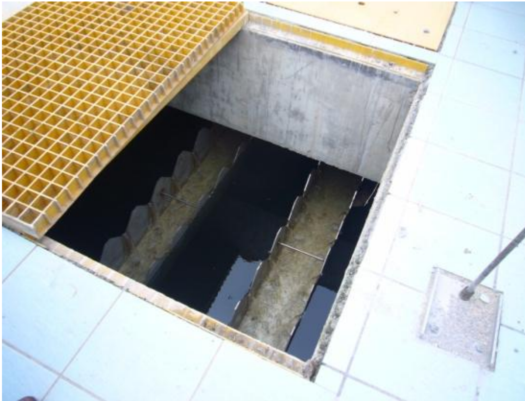
Photo 8 Secondary sedimentation tanks are covered by plastic covers
