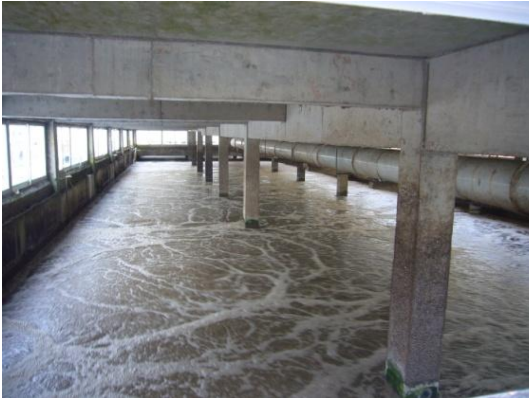
Photo 4 Biological treatment tanks are enclosed by windows
