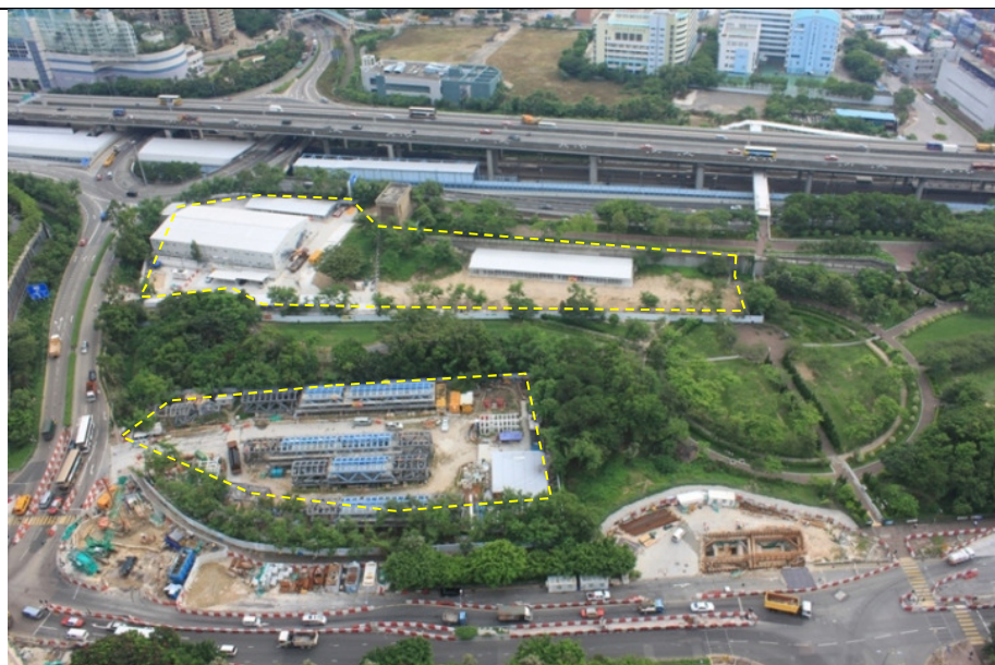
LR 4-3 Bounded by Sham Mong Road and Lin Cheung Road, inside Nam Cheong Park, as a current construction site of MTR Express Rail Line (XRL).
