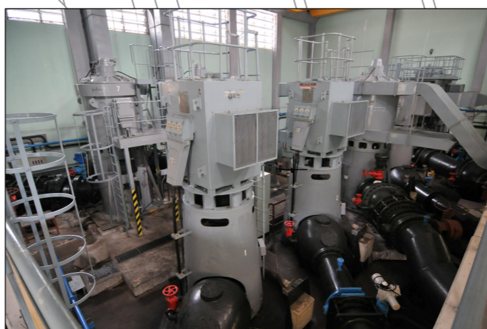
FILTERED WATER PUMPING STATION (SOUTH WORKS) (AREA A ~ 540m²)
