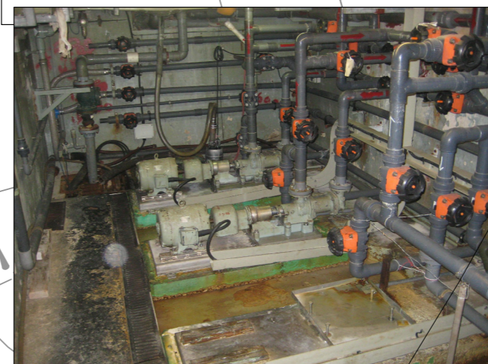
PUMP HOUSE OF ALUM SATURATOR TANK (AREA C ~ 20m 2 )
