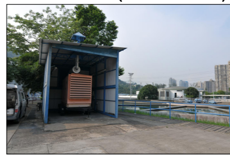
GENERATOR SET (AREA D ~ 30m²)
