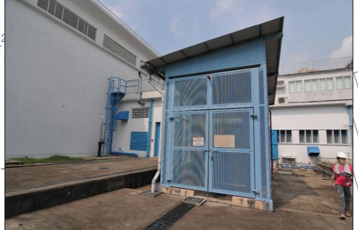
TRANSFORMER (AREA I ~30m 2 )
