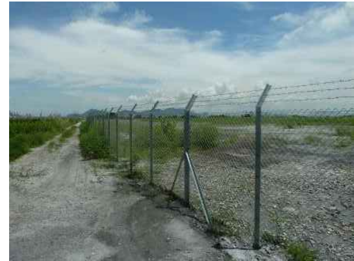
A - NARROW WATER CHANNEL ON THE WEST OF THE PROJECT SITE FILLED AND ERECTION OF A BOUNDARY FENCE
