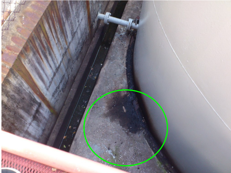
Photo 1 Stains on the Surface
