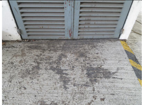
Photo 12: Stain at the entrance of the Storage Room for Chemical Waste
